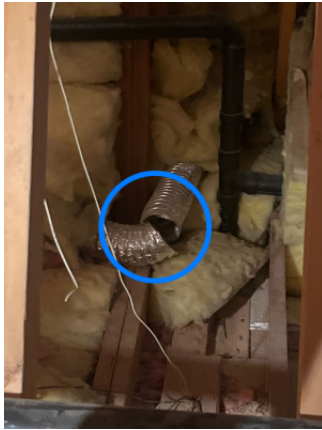
Image 8.3.1 Bathroom exhaust duct damaged
