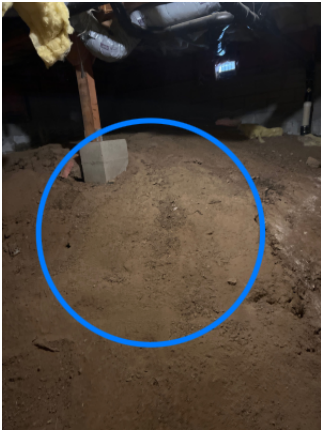
Image 8.2.1 No vapor barrier
